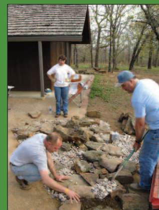
The pond liner edges were covered with large rocks, and decorative river rock was used to fill in the gaps. A garden hose soon filled the hole with water once this step was finished.
