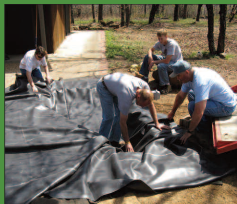
Rubber pond liner was placed in the hole and trimmed to size, leaving enough overlap around the edges to accommodate some rocks and hold it in place.
