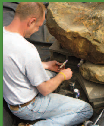
Cinder blocks formed a stable support for the bubbler rock within the hole. PVC fittings and flexible hose were used to connect the submersible pump to the hole in the bottom of our bubbler rock.
